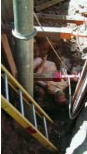
This is about a yard of soil dumped on top of a dummy. We vacuumed it up in less than 10 minutes. The vacuum truck is impressive because it sucks up large clumps of dirt and softball-size rocks with no problem.
